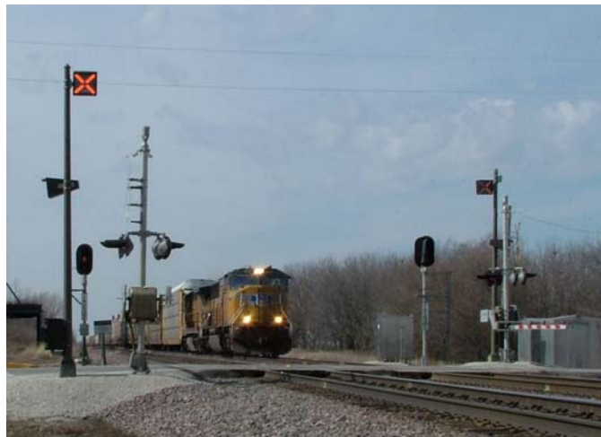
Figure 6. Example of a Wayside Horn Installation
