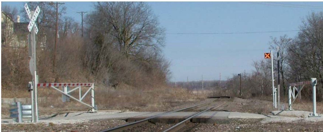
Figure 7. Example of a Temporary Closure System
